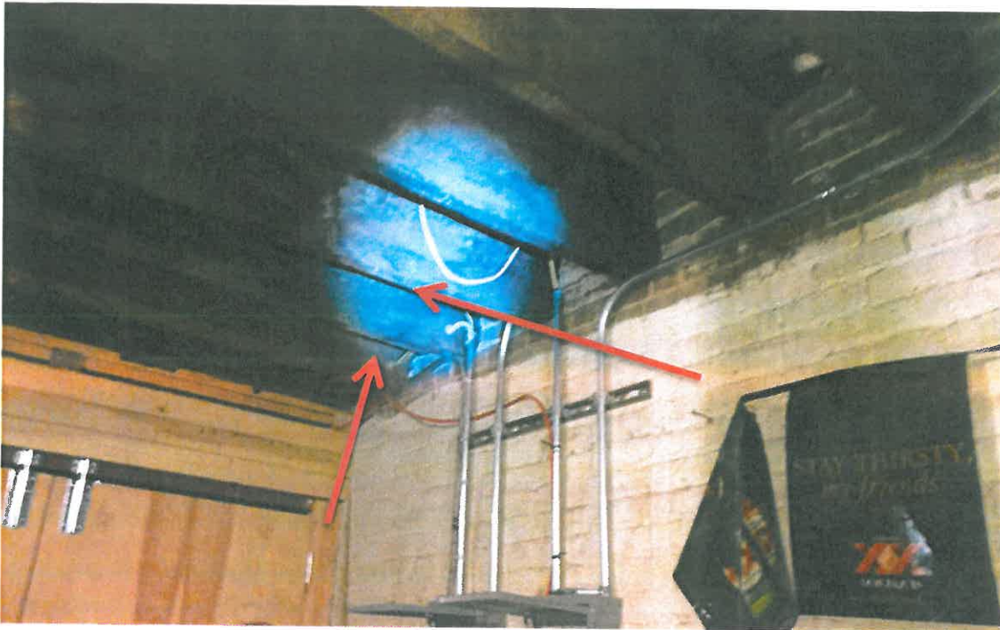
In Basement Electrical Wiring
