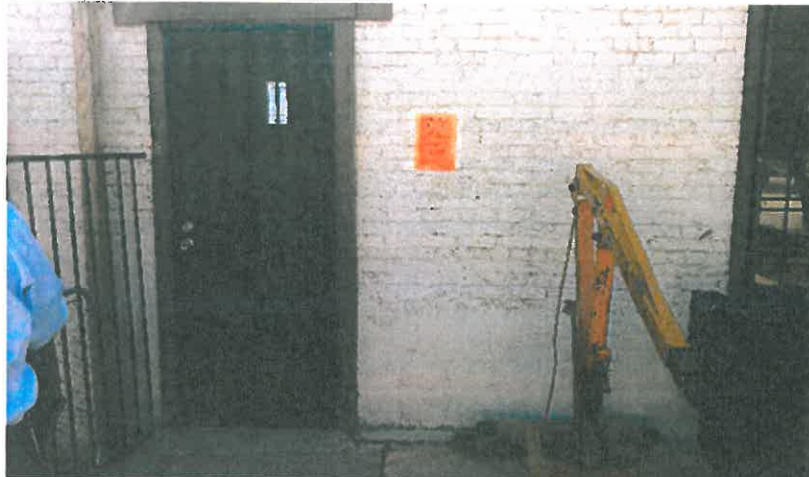
Dangerous Building Posted on 3/16/17
