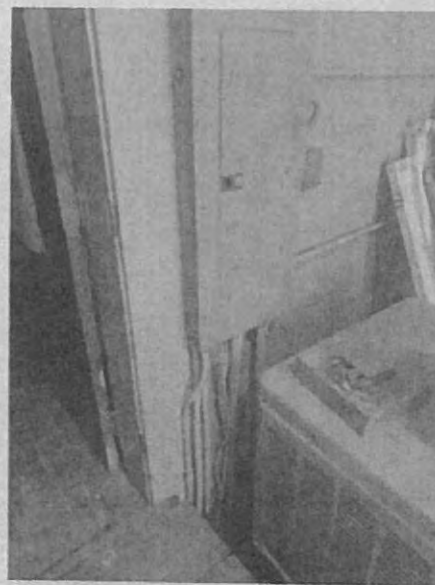
Panelboard, garage area (conflicts with evaporative cooler)
