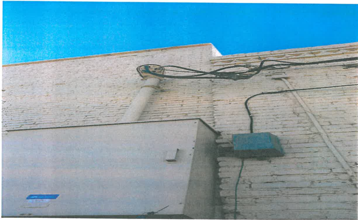
Electrical Service Box
