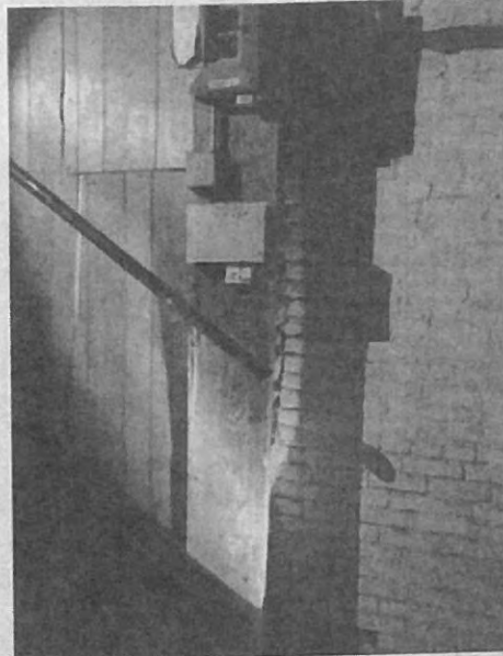
Basement 1 Panelboard, steps leading to basement
