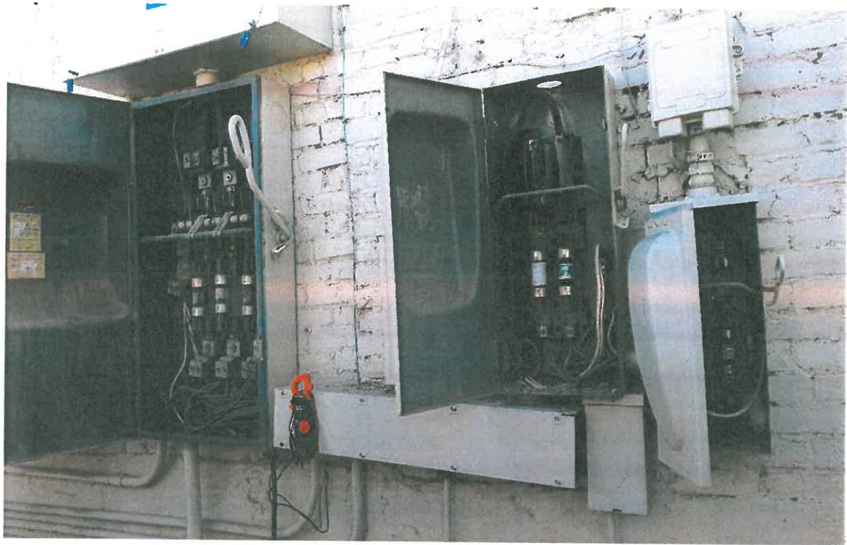
Electrical Service Box (Weather Head)
