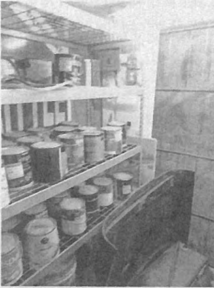
Small load center in hallway, near west door (conflicts with shelves)
