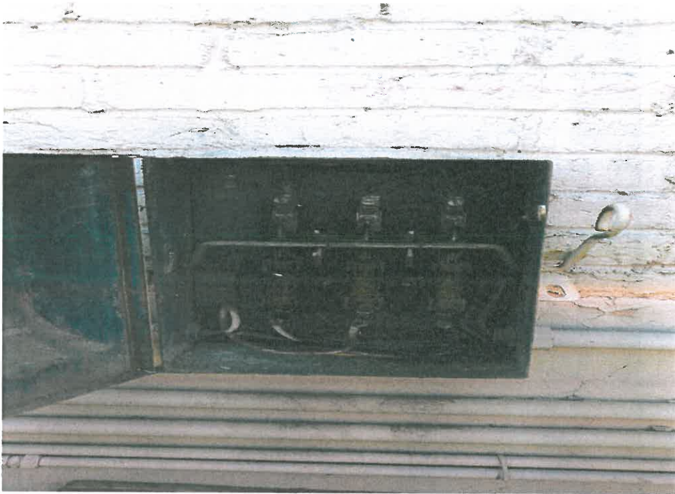
Electrical Service Box
