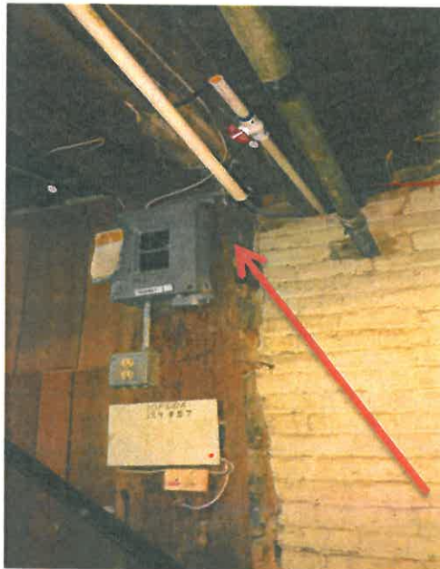
In Basement Electrical Wiring Leading out of West Basement Exit
