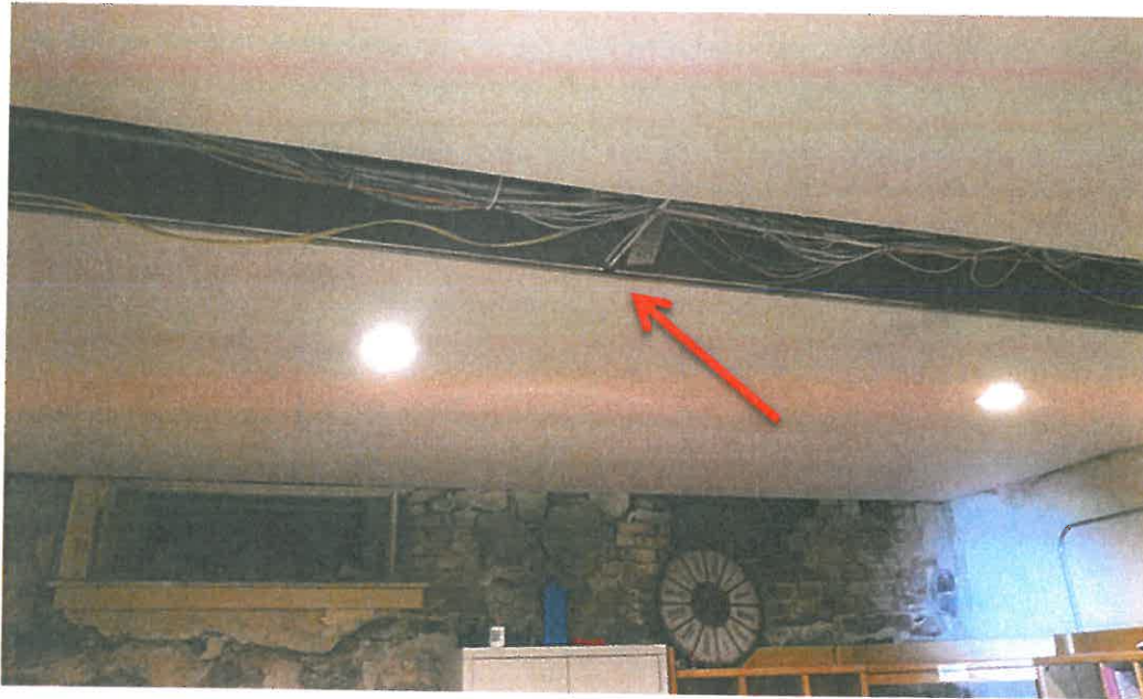
Low voltage Wire Chase between trusses
