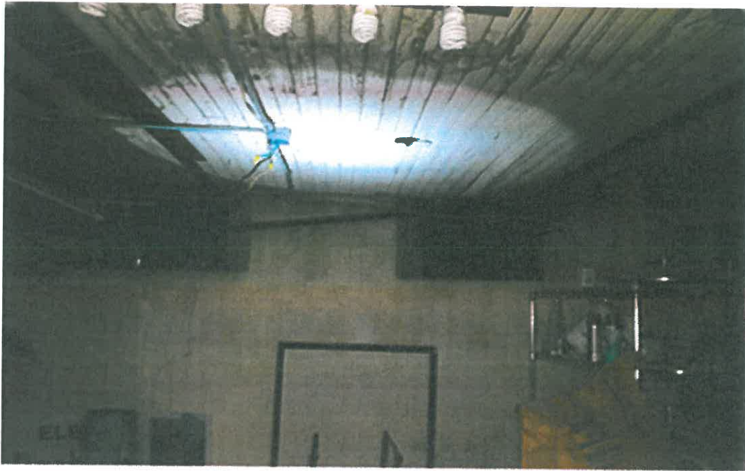
In Basement Storage Exposed Wiring and open junction boxes
